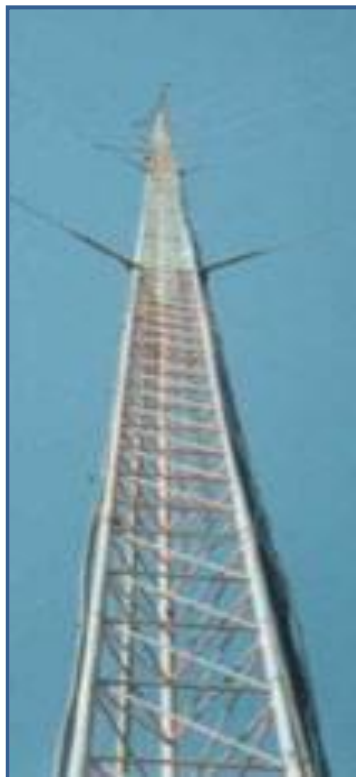
Non-Compliant Paint (FCC)
