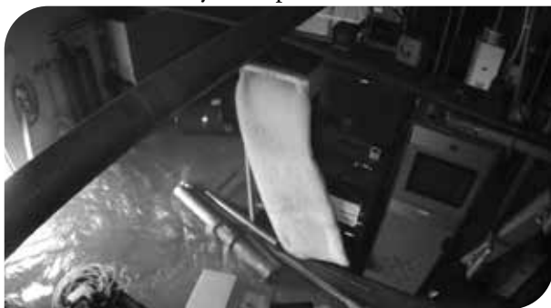
This site's equipment was destroyed by Hurricane Ian. Courtesy of John Clark, Relevant Radio
