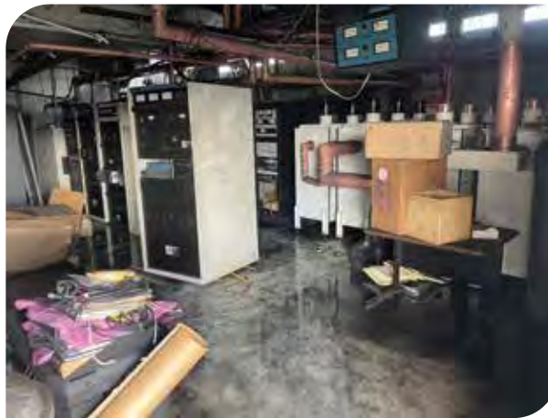
After a fire, smoke and water damage can be more extensive than the fire damage.
