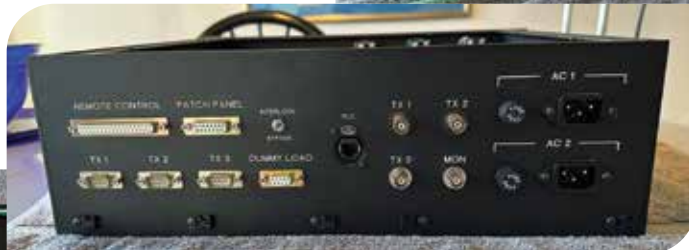
The front panel, rear panel, and interior of Lynn's PLC transmitter controller.
